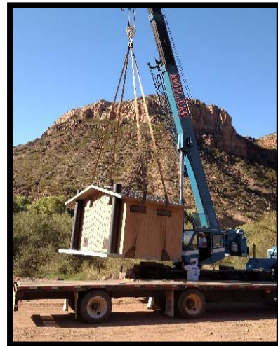
Restroom delivery on San Francisco Road
